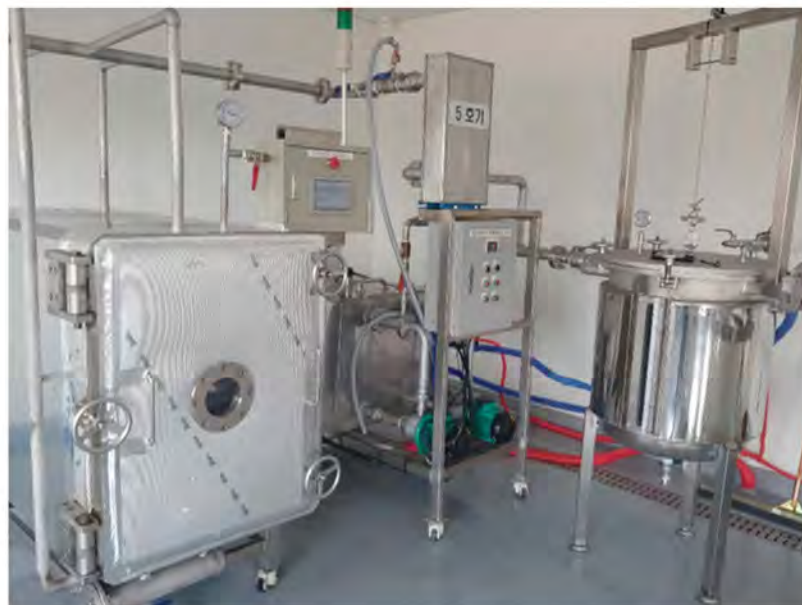
Fig. 13 Vacuum dryer installed in Lava Seawater Complex
